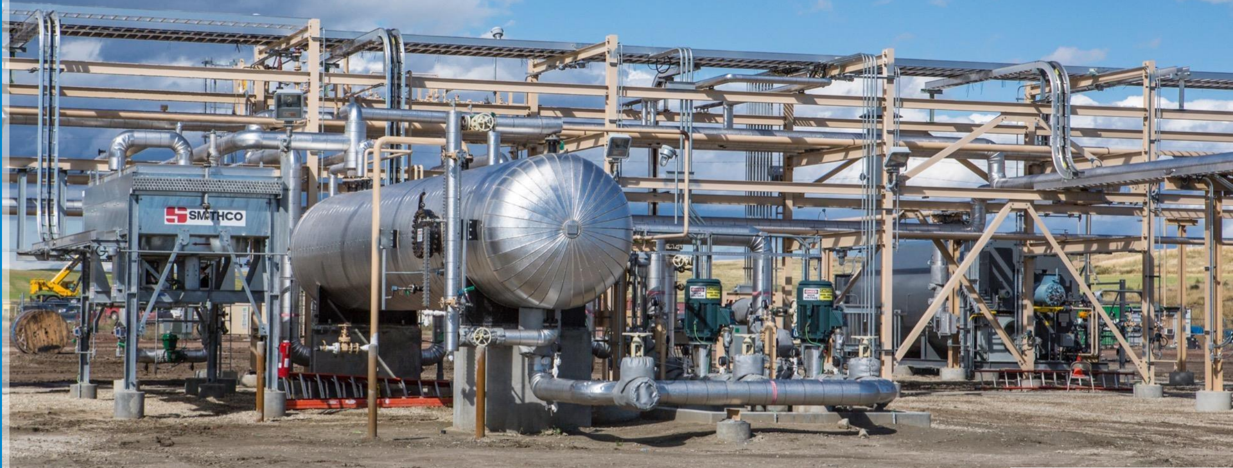
Bear Creek plant — Williston Basin
