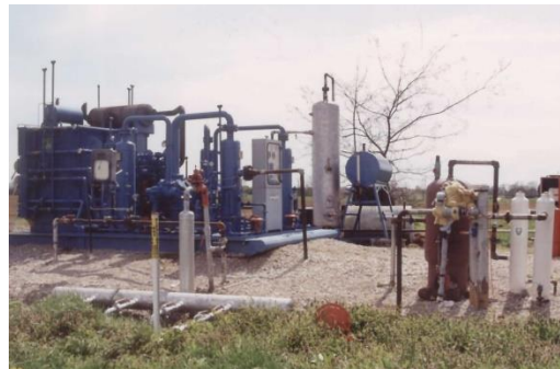
Compressor Station with Desiccant Dehydrator
